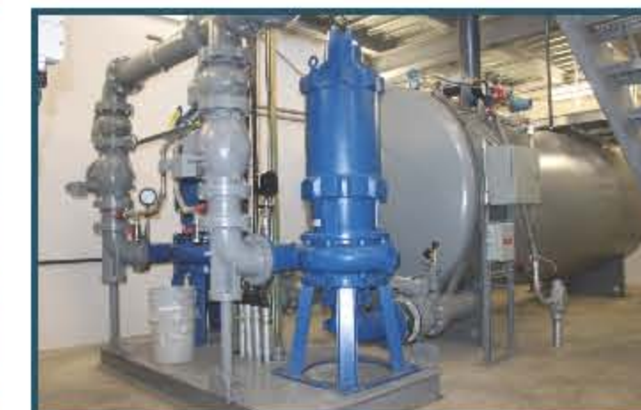
7. Installed sewage pumps and piping in lower level of pump station
