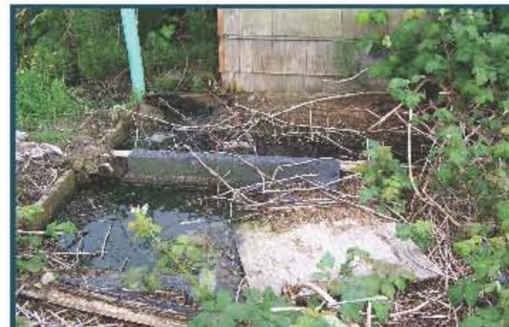
1. The problem: Failed septic systems
