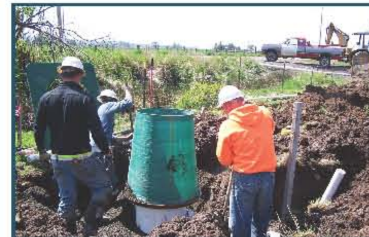
2. Installation of a valve pit that typically serves up to four homes
