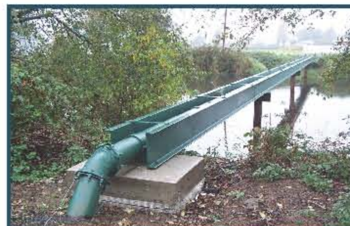
5. Vacuum pipe and pipe bridge over Jeffers Slough
